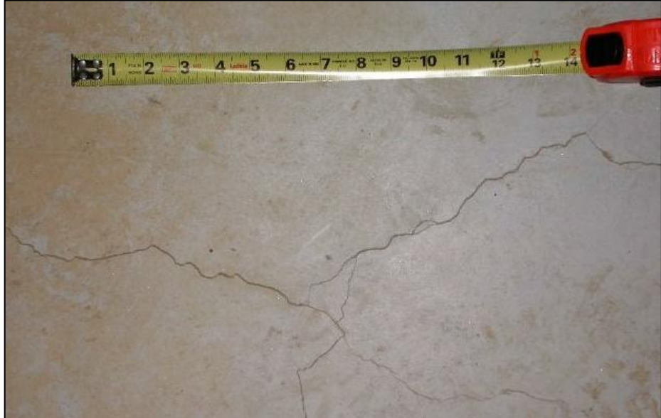
Figure1.9 Minor cracks on floors of ground floor
